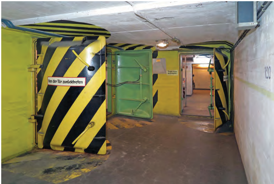
The restored and fully-operational hydraulically-operated blast doors at Steintorwall Bunker. In the centre of the far wall can be seen the small window which connects to the control room. The placard is an invitation to keep fingers clear
